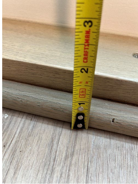
Figure 1: A threshold to the outdoor patio in Unit 116 measuring above 3/4 inches without a sufficient bevel
