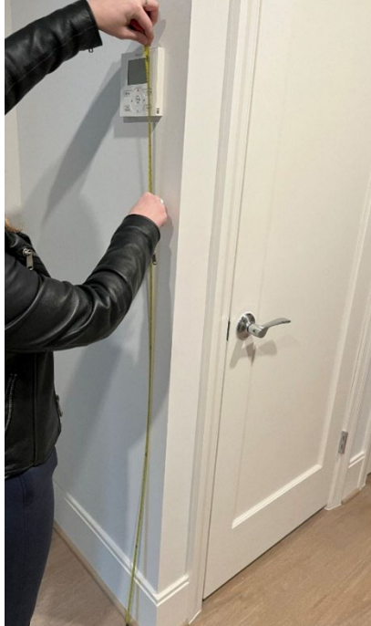
Figure 5: Unit 430's thermostat with operable parts at approximately 57 inches
