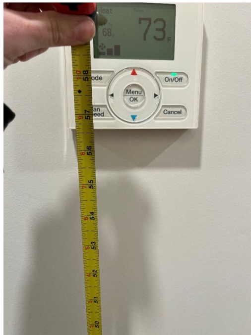
Figure 6: Unit 412's thermostat with operable parts at approximately 57.5 inches
