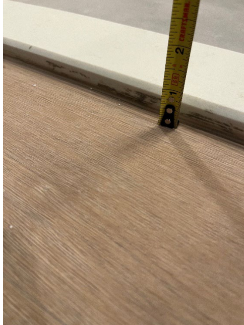
Figure 4: Unit 430’s bathroom threshold measuring above 1/4 inch without a sufficient bevel
