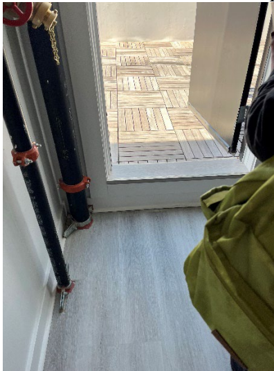
Figure 1: Interior threshold at entry to rooftop deck.
