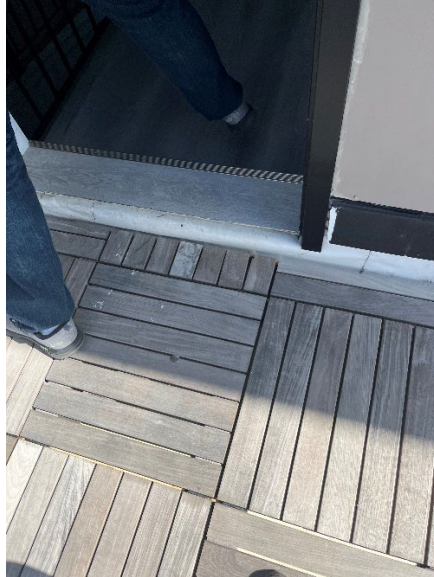
Figure 2: Exterior threshold at entry to rooftop deck.
