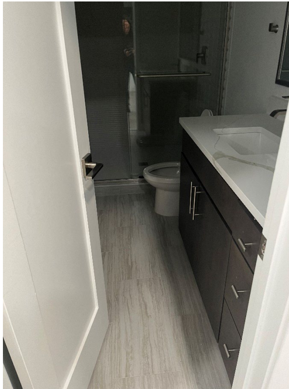
Figure 16: Unit 302 bathroom featuring less than 30" x 48" of clear floor space.
