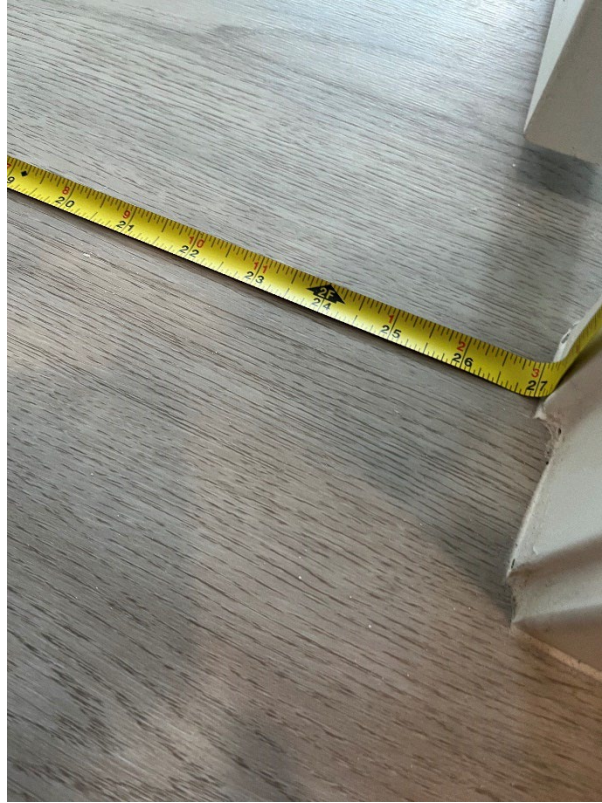
Figure 3: Unit 409 bedroom door measuring approximately 27 inches.
