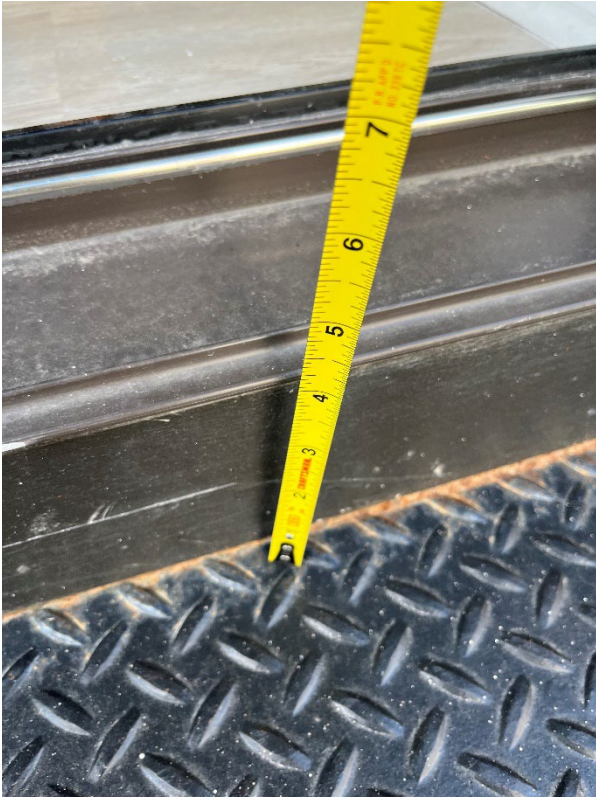
Figure 11: Unit 409 secondary exterior door threshold measuring 5 inches.
