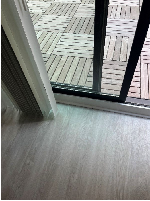
Figure 10: Unit 302 secondary exterior door threshold measuring in excess of 1 inch.
