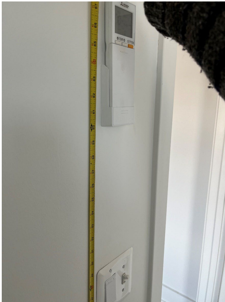
Figure 12: Unit 411 temperature control device mounted above 60 inches.
