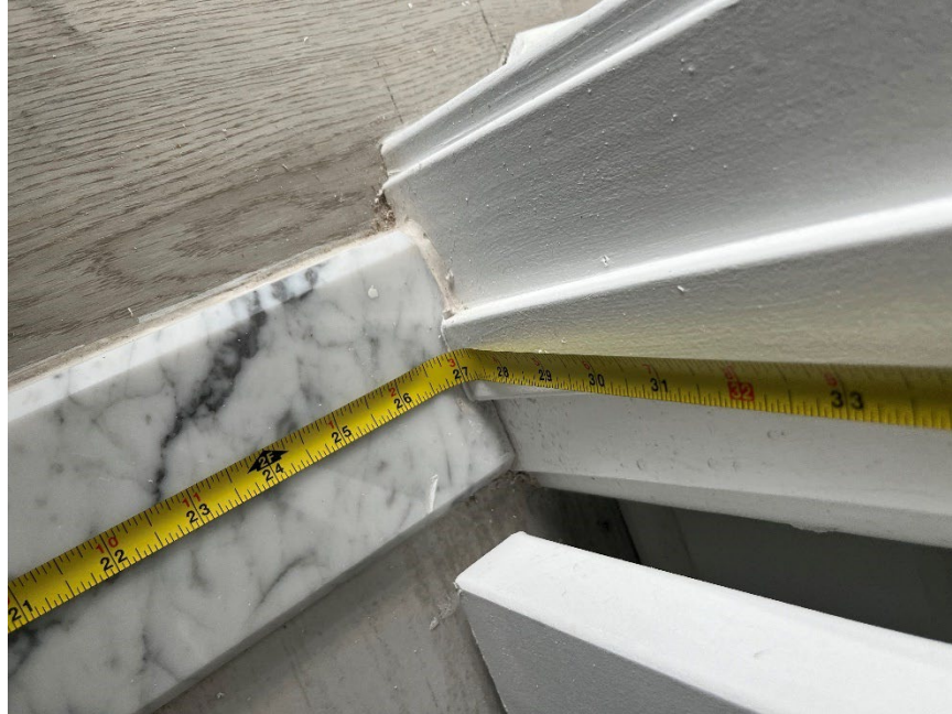
Figure 7: Unit 411 bathroom door measuring approximately 27 inches.
