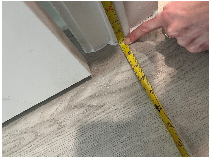
Figure 4: Unit 302 bedroom door measuring approximately 29 inches.
