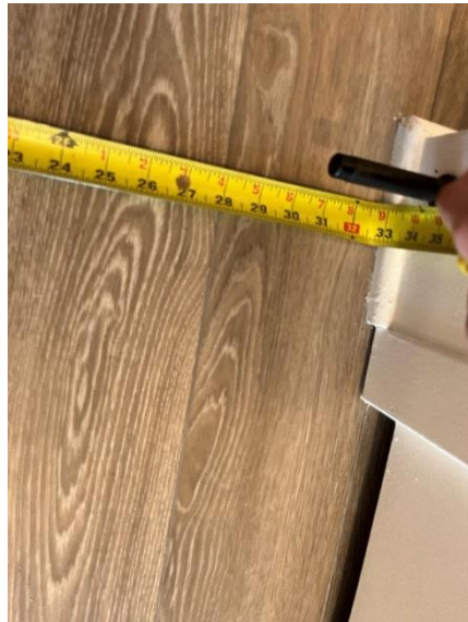
Figure 5: Unit 204's hallway narrowed to 33 inches.
