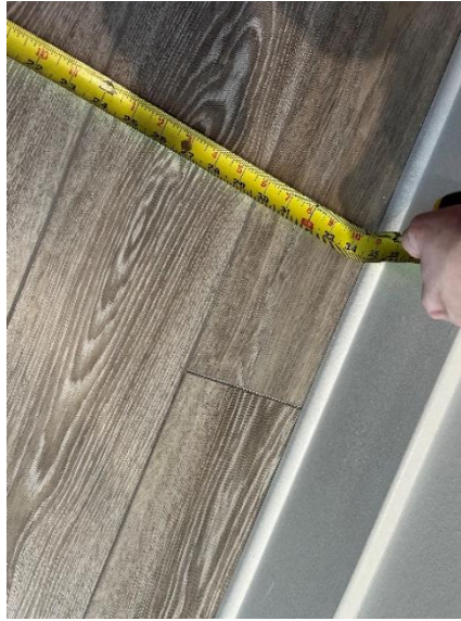
Figure 4: Unit 302’s hallway narrowed to 34 inches.
