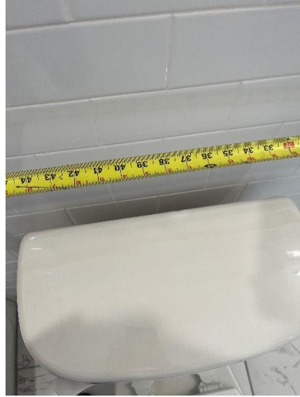
Figure 2: Unit 302 toilet centerline of approximately 38 inches.
