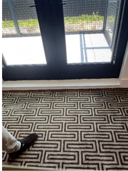
Figure 7: The rooftop deck's estimated unbeveled interior threshold was at least four inches.
